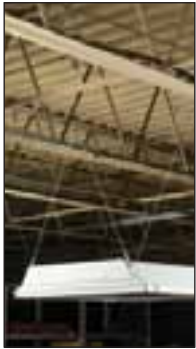
High Bay Lighting
